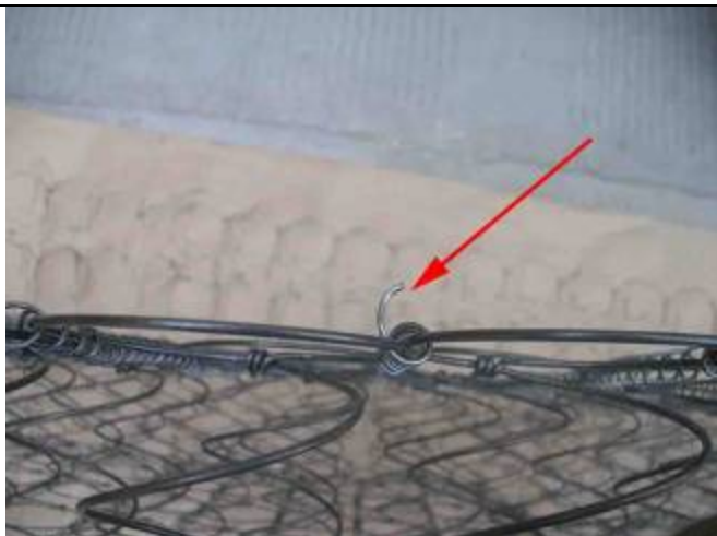
c.1. the Helical wire head was fixed improperly
